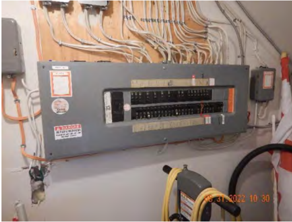
Figure 4: Lower Level Panelboard
