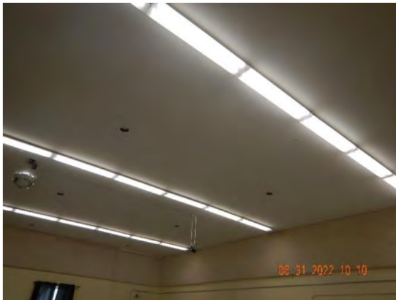
Figure 7: Multipurpose Room Lighting
