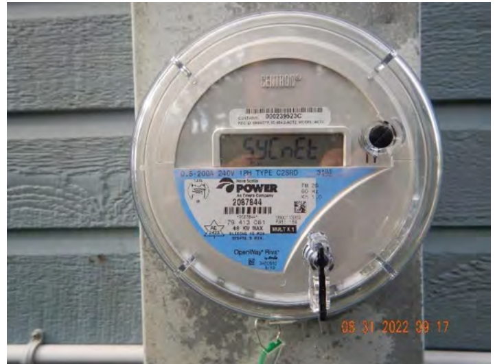
Figure 3: Lower Level Meter
