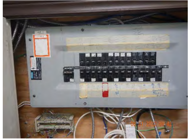
Figure 5: Upper Level Panelboard
