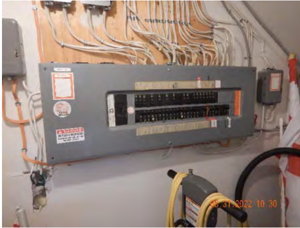
Figure 4: Lower Level Panelboard
